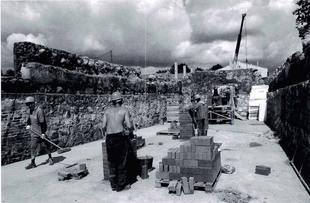
Preparing the walls for the future storage houses of the Estonian National Museum. Photographic collections of the Estonian National Museum. Photo by Arp Karm.
